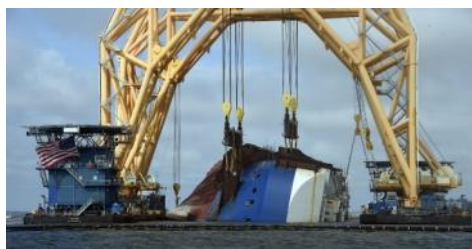
Anchor chain attached to the pulley system on the VB-10000 heavy-lift vessel moves slowly to cut through Section One of the Golden Ray wreck. St. Simons Sound Incident response photo.
